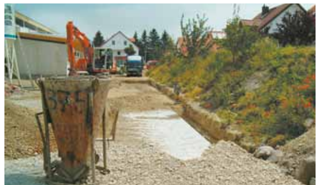
Laying the covering layers in the front-dumping method to allow vehicles to drive on the structure.
